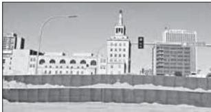
A flood wall made of Hesco barriers lines the banks of the Cedar River in Cedar Rapids, Iowa, on Monday.
