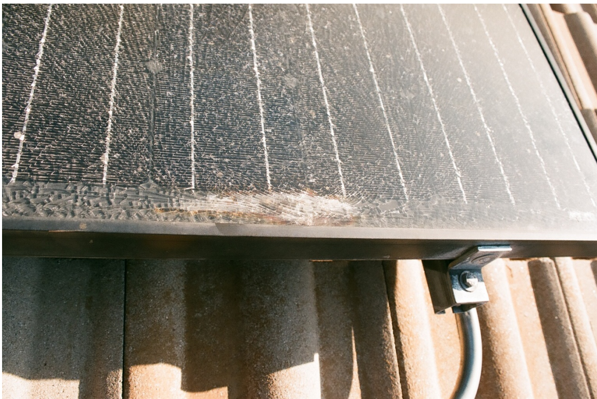
Model No. BP 4175B (Allagas Property) Burn Mark and Shattered Glass from Junction Box Failure
