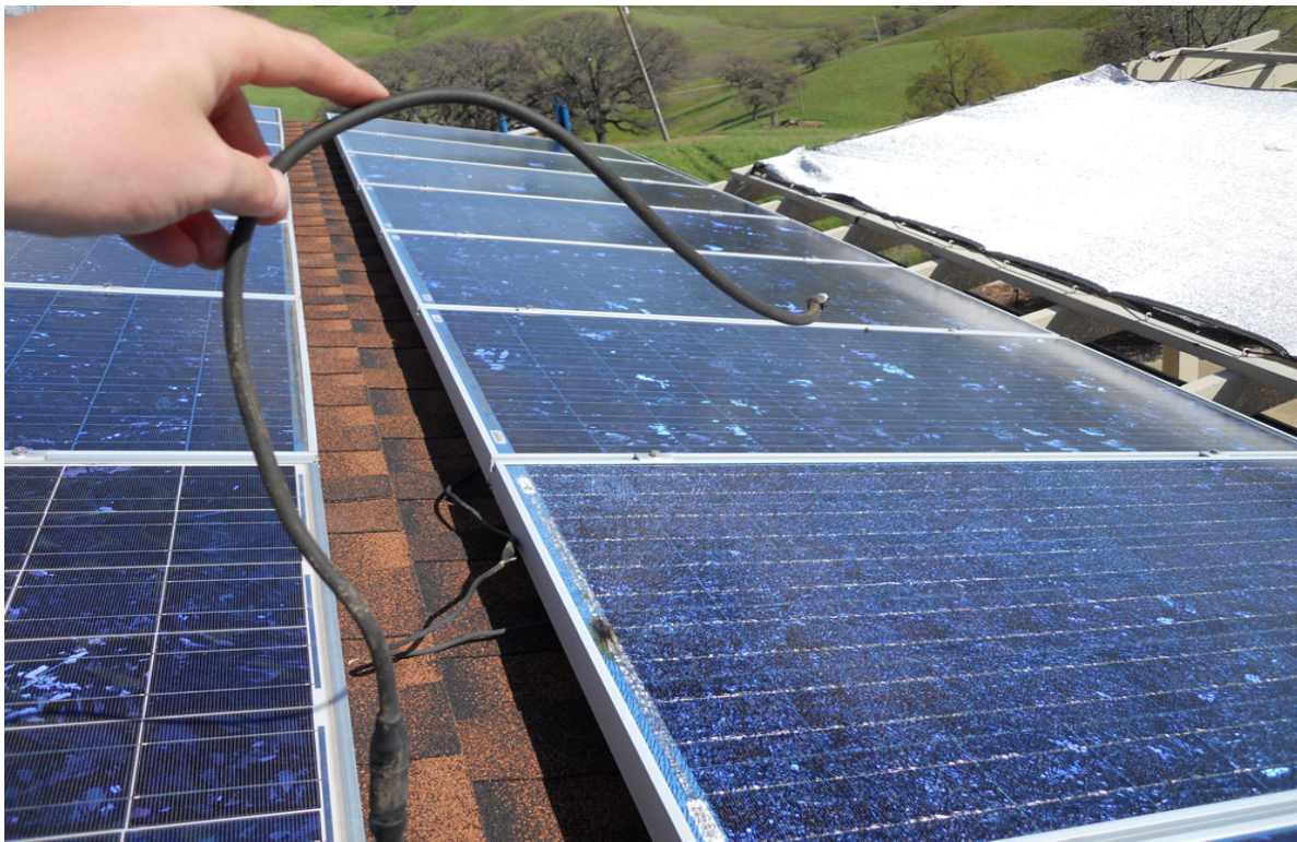
Model No. BP SX3 150S – Burned Connecting Cable Associated with Junction Box Failure
