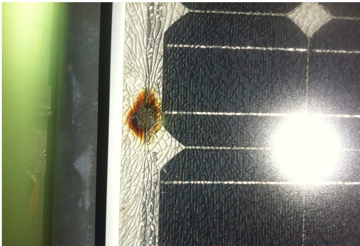
Model No. BP 2150S (Mohrman Property) Burn Mark and Shattered Glass from Junction Box Failure
