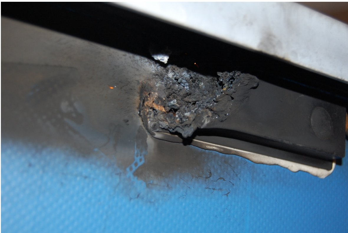
Model No. BP SX3 150S (Back) Melted junction box due to overheating caused by junction box failure.
